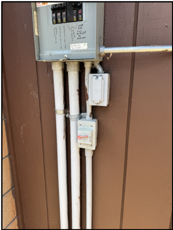
2 E103 VIEW OF PANEL, RECEPTACLE, AND SWITCH
