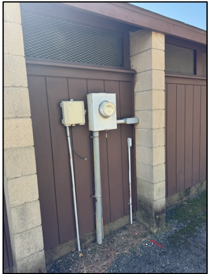
3 VIEW OF METER AND TELECOM BOX E102
