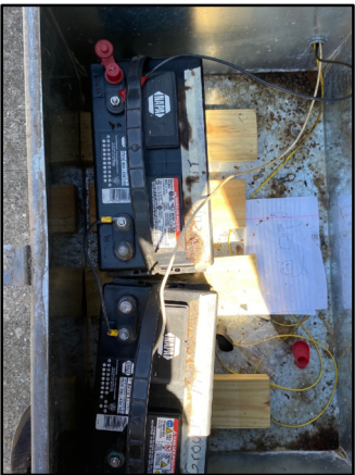
3 E104 VIEW OF BATTERIES FOR SOLAR
