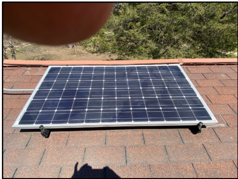
6 E104 VIEW OF ROOF MOUNTED SOLAR PANEL
