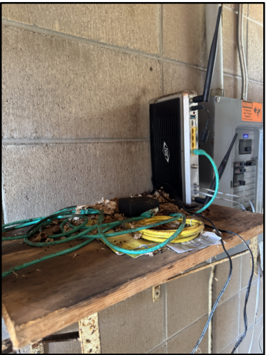
4 VIEW OF PANEL AND DISCONNECTED ROUTER E102
