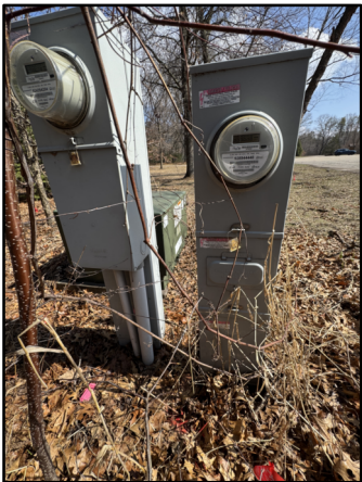
3 E103 VIEW OF UTILITY METERS
